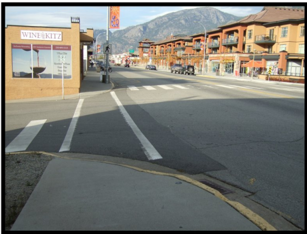
Photo 91: Steep curb ramps along Main Street
