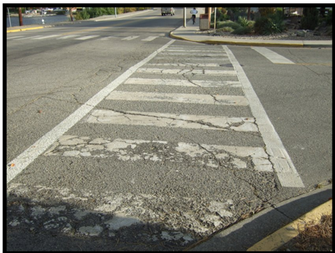
Photo 86: Cracked pavement at Kingfisher Drive crosswalk (by Veteran's Park)
