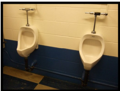
Photo 25: Sun Bowl Arena – Urinal in men's washroom
