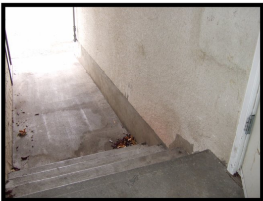
Photo 40: Planning and Development Services – Hazard at top of ramp
