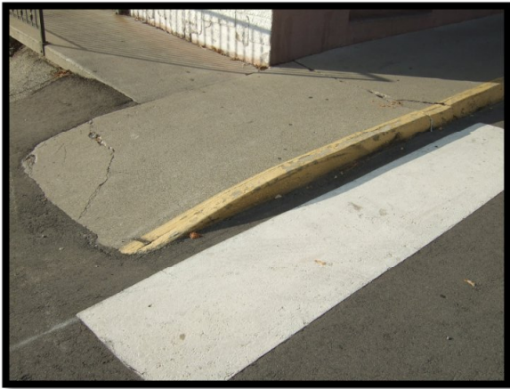
Photo 90: Steep, inaccessible curb ramp by Pizza Factory
