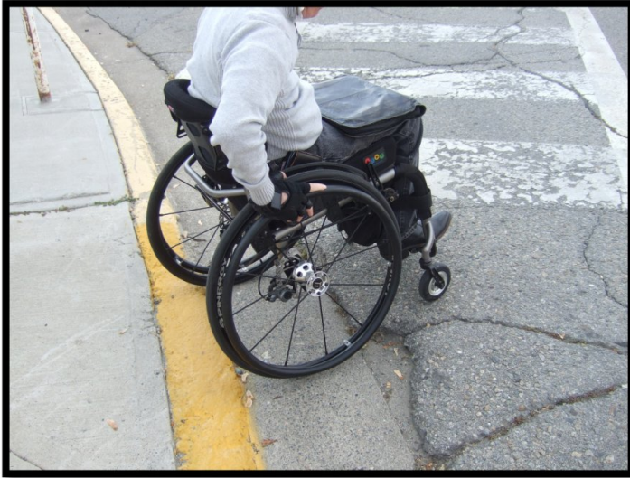
Photo 88: Cracked pavement at crosswalk at 68th Ave and Main Street
