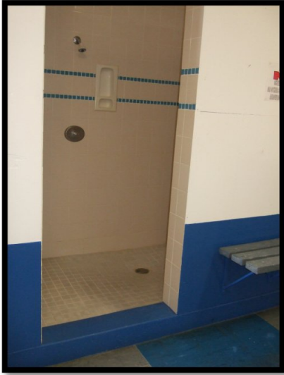
Photo 30: Sun Bowl Arena – Example of inaccessible washroom stall in change room
