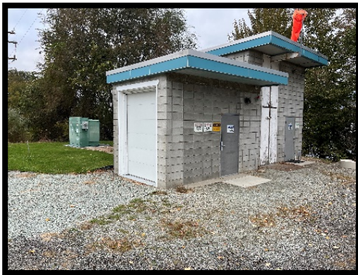
1*Picture of Station #8 lake intake.
